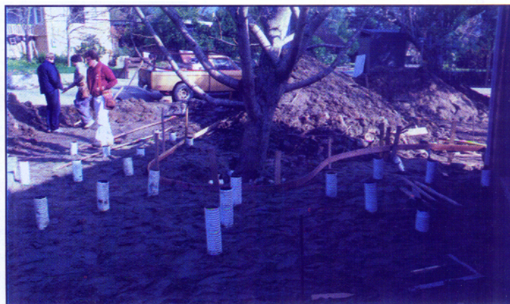
Figure 5. Aeration systems often are specified to counteract a perceived aeration deficit that follows a fill event. Here, multiple vertical aeration pipes are connected to underlying horizontal pipes that radiate out from the tree base. Although this system is thought to improve aeration status in the root zone, research has not supported a positive impact of similar systems on oxygen concentration or oxygen diffusion rate in the root zone.
