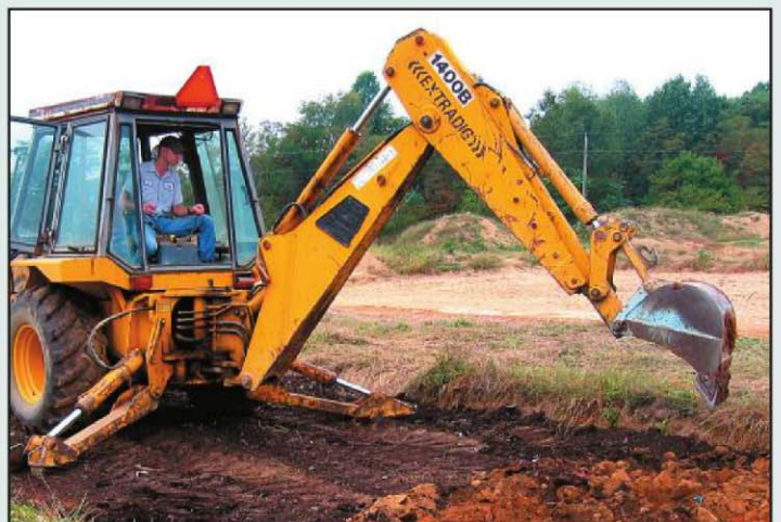
This photo illustrates the “scooping and dumping” subsoiling process in Soil Profile Rebuilding. Compost laid on surface is being incorporated 2 feet (.6 m) down with backhoe. Photo by Rachel M. Layman, former MS student who installed plots for the study.
